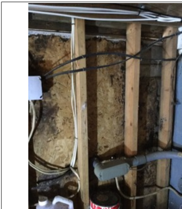
Some moisture stains
