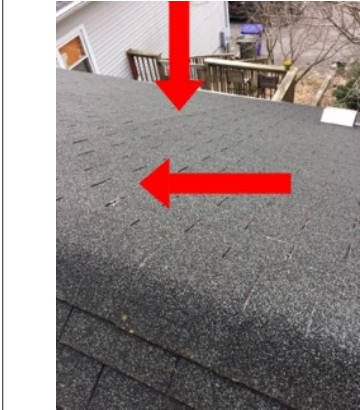
Slight ridge here and a few soft spots. As long as the shingles are ok a little soft spot can be repaired when the roof is redone in the future.
