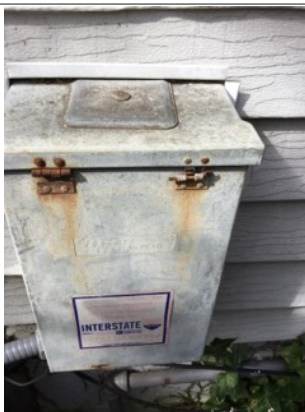
Door hinges are broken on electric breaker box
